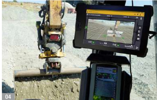
Abb. 04: Screen Trimble Earthworks [SITECH]
